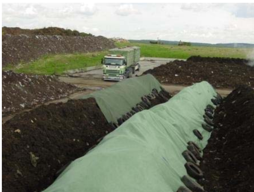
Covered windrows, left side Ten Cate Nicolon, right side Polyfelt
